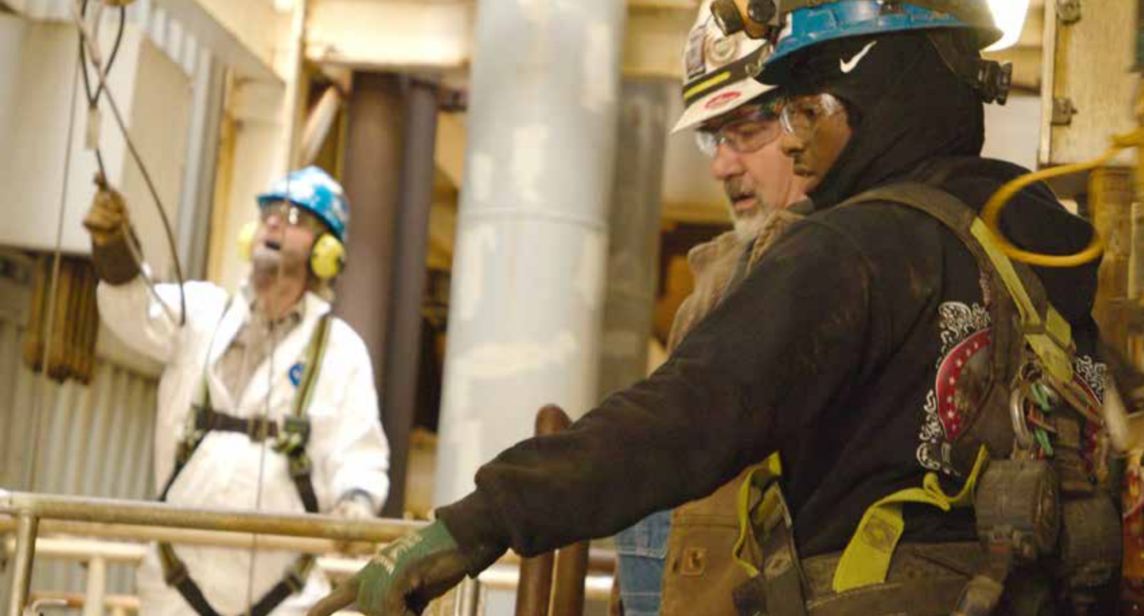
L-455 Boilermakers rig at TVA's Cumberland Fossil Plant. L to r: Barry Breece sets up in the background while journeyman Dan Gray instructs apprentice Reginald Lewis.
