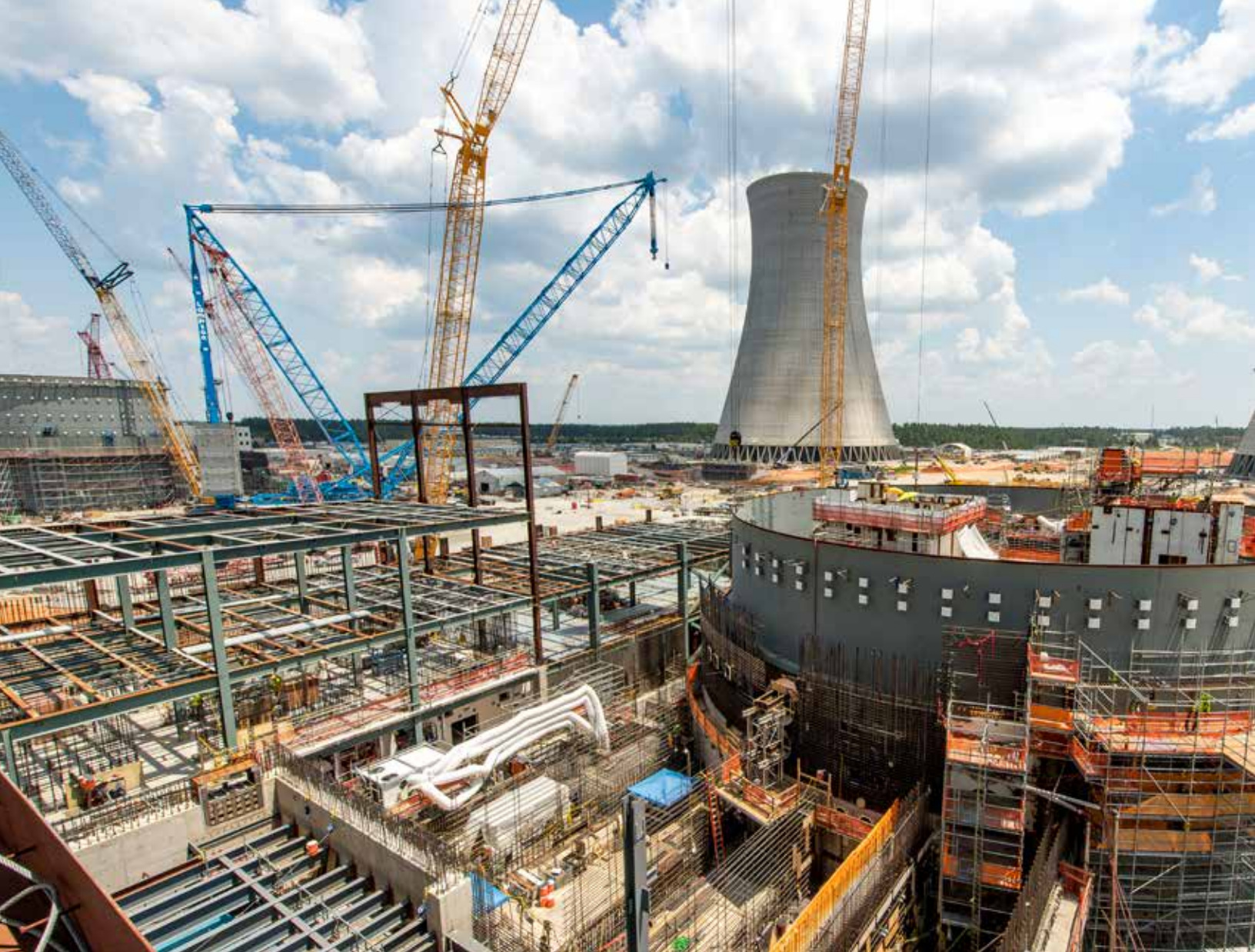
Boilermakers were instrumental in building Plant Vogtle, with Units 3 and 4 (pictured above under construction in 2019) completed in 2024.
