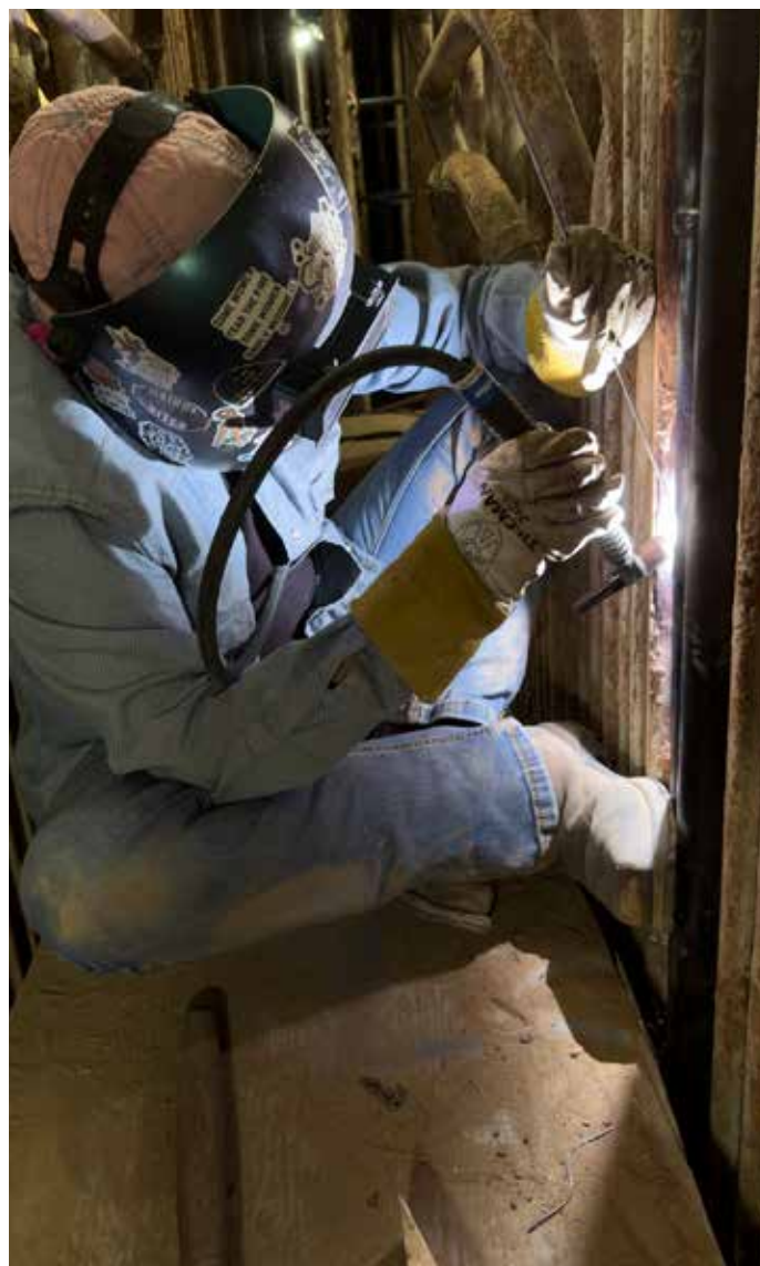
Gregory wedges herself in to get the job done. She has already earned a solid reputation as a dependable Boilermaker sister.
