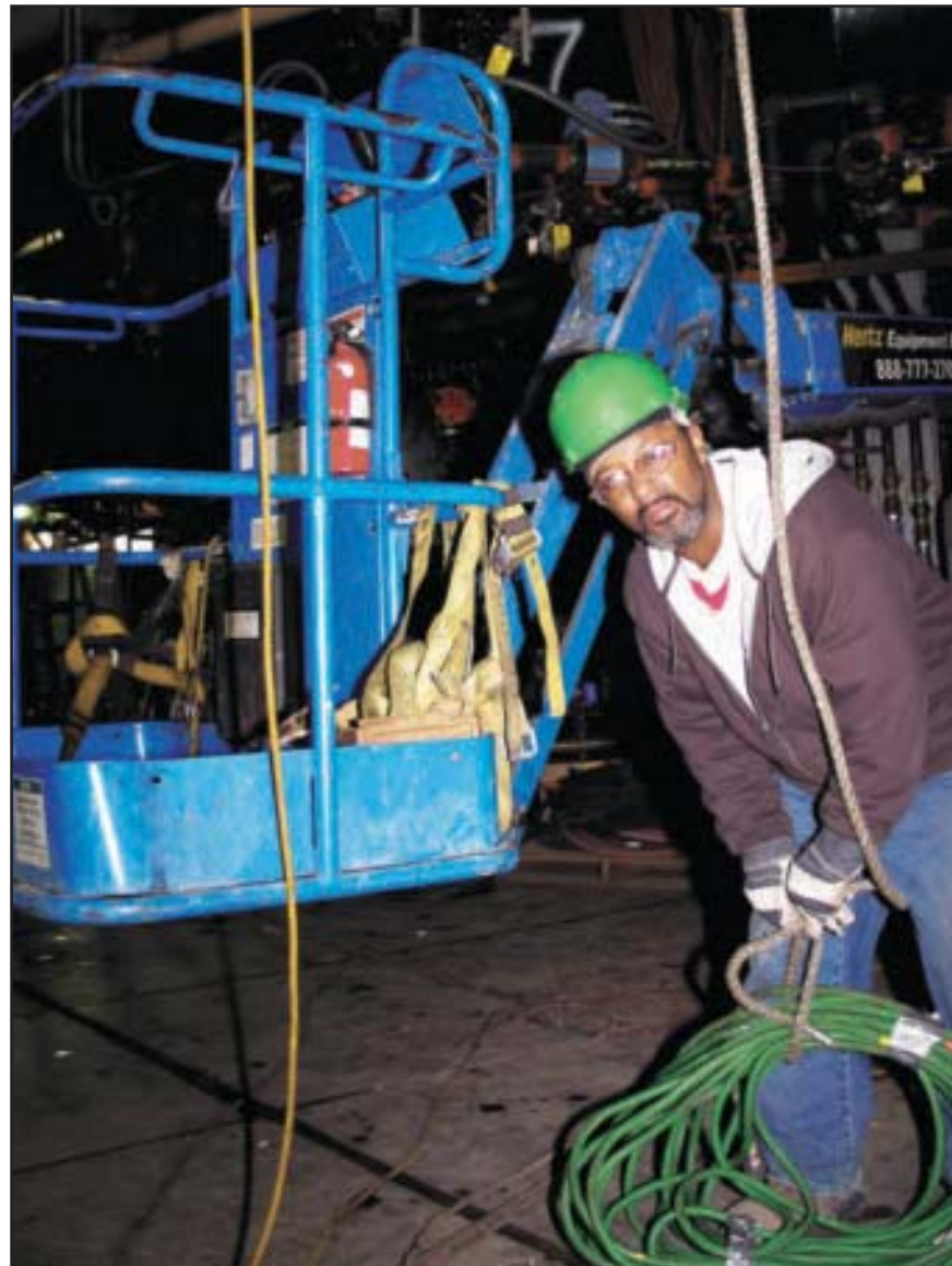
L-169 member Terrence Coursey unravels a welding lead as it is lowered from the new SeverStal "C" blast furnace.
