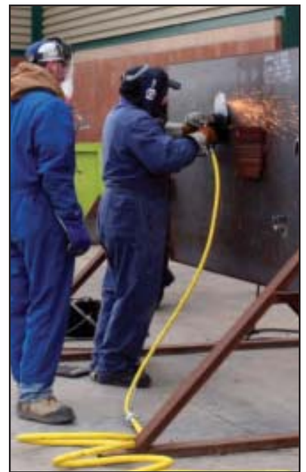
Students of the L-146 WorkSmart program experience the physical demands required of a Boilermaker while working with nine-inch grinders.
