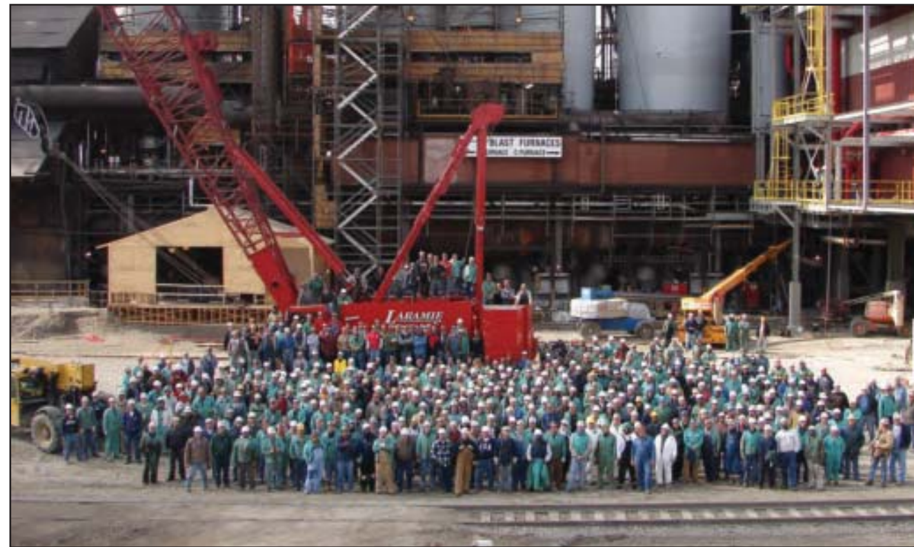
Here is part of the building trades and contracting crew (including members of Detroit Local 169) that set a new industry standard by installing a "C" blast furnace in less than 100 days at SeverStal North America's Ford Rouge site.
