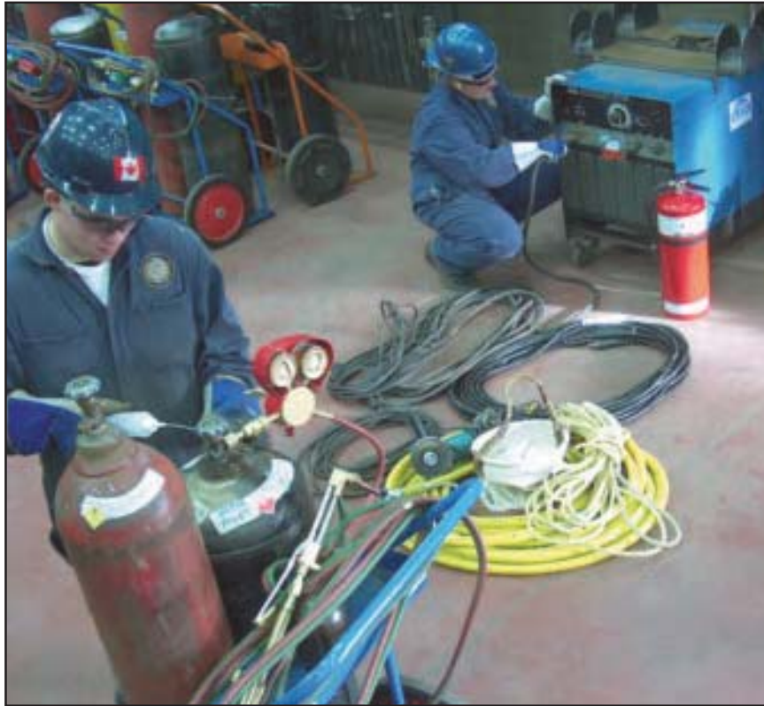
Hands-on training at the Local 146 WorkSmart program includes learning how to safely set up and use oxy-acetylene cutting equipment.
