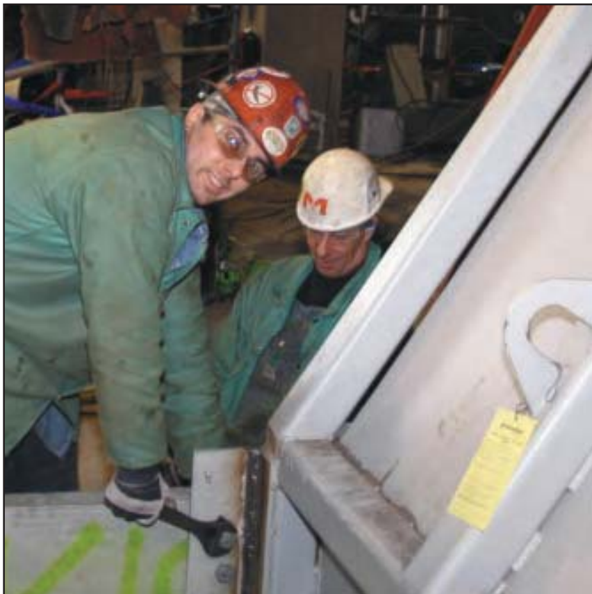
Putting a wrench to an emissions duct hood at the SeverStal "C" blast furnace are L-169 members (l. to r.) Darryl Coch and Tom Hamilton.
