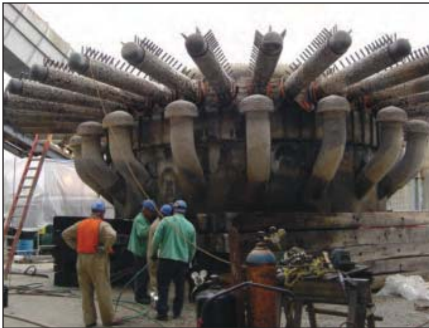
Local 40 members finalize the removal of the regenerator's old air grid at Marathon Petroleum.
