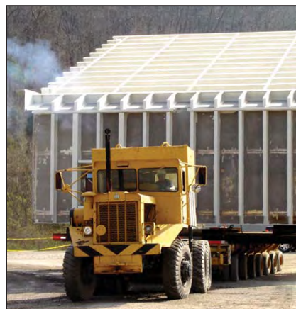
L-453 Boilermakers will need 125 truckloads of structural components to complete work at TVA's Bull Run fossil-fuel power plant near Knoxville, Tenn.
