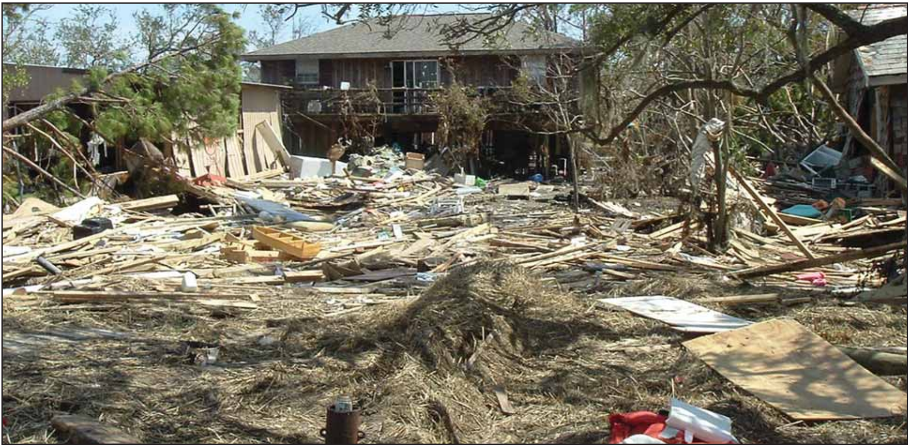
Hurricane Katrina not only damaged homes, it obliterated many, leaving only piles of sticks and trash.
