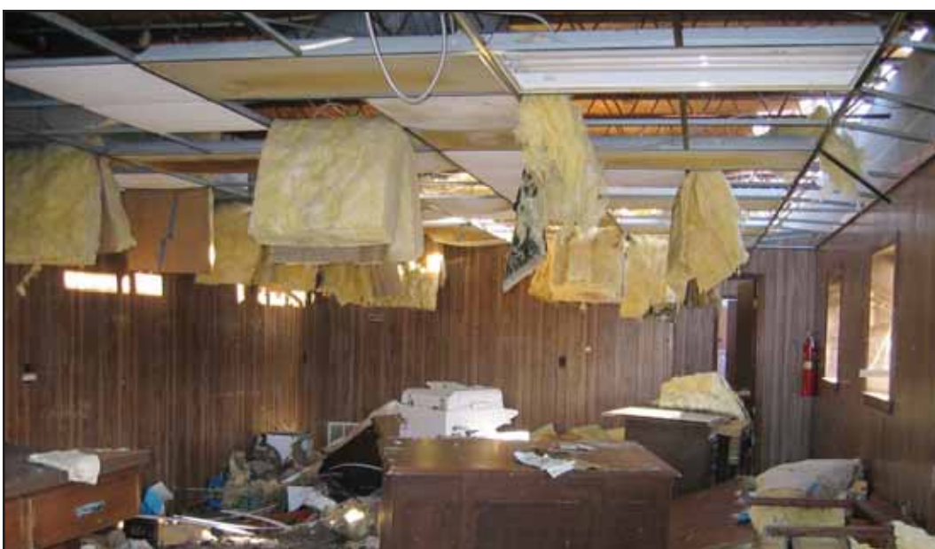
The roof of Local 693's hall gave way, destroying nearly everything inside.
