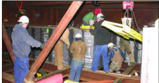
IN THE BOWELS of the selective catalytic reactor, Local 169 members install a series of catalyst blocks, which weigh a ton each. (Source: The Building Tradesman )
