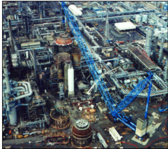
LOCAL 28 MEMBERS use the world's largest crane, a Lampson LTL-2600, to complete Nooter Construction Co.'s largest single lift ever — 704 tons at a 287-foot radius — while working a turnaround at a ConocoPhillips refinery in Bayway, N.J.
