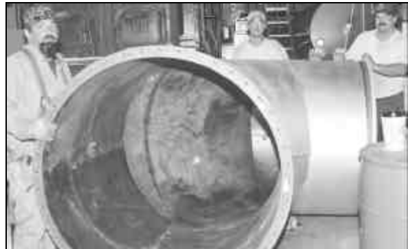
WORKING FOR WOODLEY-Griggs Boiler Repair LLC, these Local 83 members, Kansas City, Mo., are replacing 54-year-old ductwork at International headquarters in Kansas City, Kan. Pictured, l. to r., are Chris Kattou, apprentice Nick Scherman, and John Malone. □
