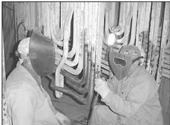
TWO LOCAL 83 MEMBERS, Mike Hendrickson (l) and Bobby Dill (r), add new super heat element loop tubes at the Nearman Power Plant in Kansas City, Kan. Of the 1,018 welds, only 0.53 percent were rejected and those required only minor repairs.
