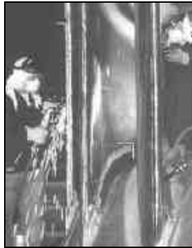
L-359 MEMBER try a new technique — hand-gouging stay ring vanes — at a hydroelectric dam in Hudson Hope, B.C.
