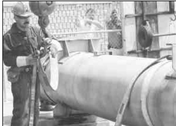
LOCAL 146'S DARREN HOFFMAN participates in the rigging exercise of the ninth annual Canadian Boilermaker Apprenticeship Competition, June 23-26, 2002.
