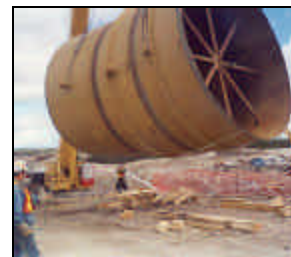
L-203 MEMBERS prepare to lower one of the penstock sections into place.
