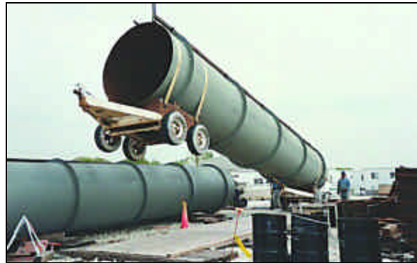
ABOVE: NTL MEMBERS use a crane and temporary wheels to help set one of 56 tube sections into place.
