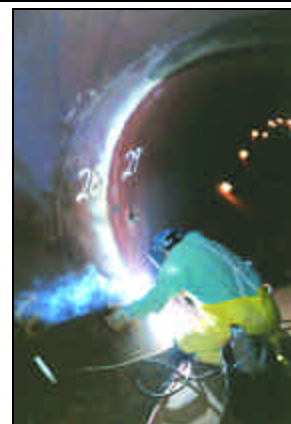
AT RIGHT: ALIGNMENT IS A CRITICAL factor as an NTL member welds together sections of a 2,215-foot long decay tube.
