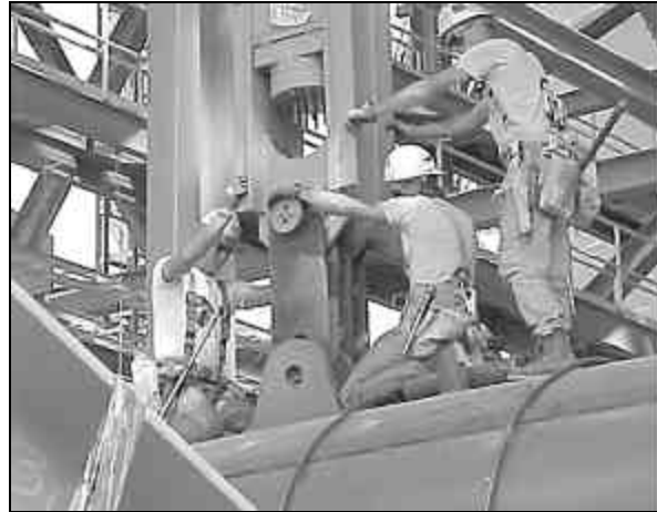
Not even Marmaduke, for whom their award is named, could have brought Hawthorn Unit 5 back from the ashes faster than the team of KCP&L, Babcock & Wilcox, and Burns & McDonnell employing Boilermakers from U.S. and Canada.
