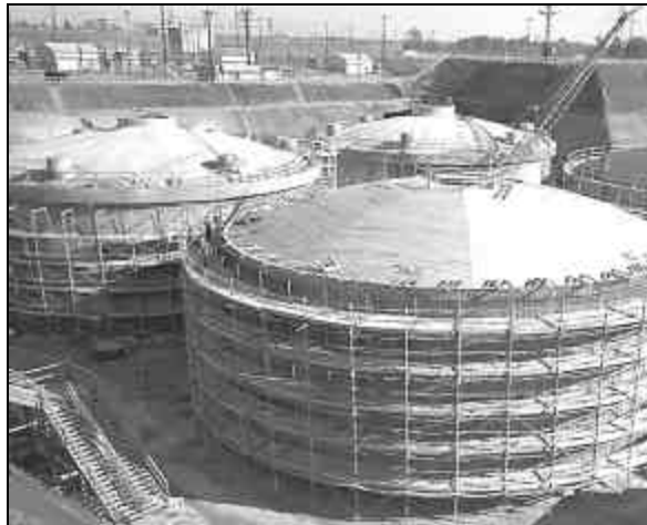
Boilermakers who worked on this Westinghouse Savannah River Company nuclear waste storage tank, shown under construction in the 1950s, are eligible for this program, as are many others who worked on other atomic weapons sites.
