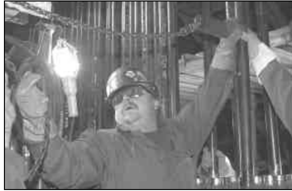
Mike Alexander, a rigger/fitter, uses a come-along while fitting a single tube during a tight-wall boiler overhaul.
