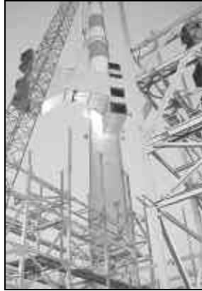
While the steam drum was being fabricated at KCP&L's Hawthorn plant, Boilermakers labored into the night through two blustery winters to erect this 550-mw boiler in reverse order.
