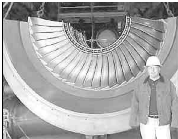
The high-efficiency steam turbine at the Klamath cogeneration project in Oregon, features advanced blading. The blades are 40-inches long and are twisted, bent, and curved for optimum aerodynamics.
