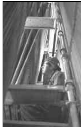
A boilermaker preps tubes for a TIG welder in a five-story boiler.
