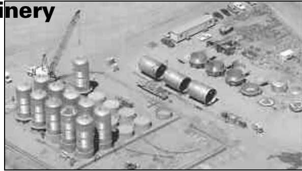
NTL members are in the process of erecting twenty 46,000-gallon fermentation tanks at the Gallo Winery in Livingston, Calif.
