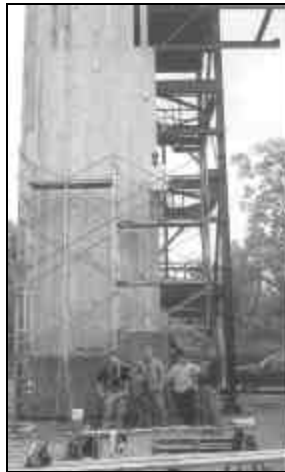
Local 7 members are building this repelling tower for the Erie County sheriff's SWAT team.
