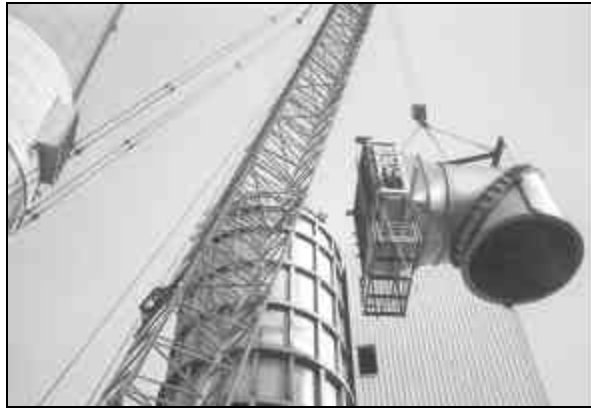
A crane lifts the absorber top, which weighs 38 tons and has openings measuring 14-foot square and 16-foot round.
