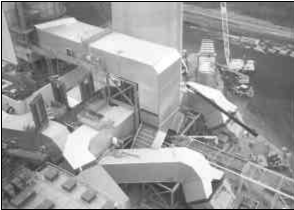
In erecting this SO 2 scrubber (shown here near completion), Local 363 members attach over 600 linear feet of ductwork.
