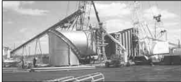
Members of Local 363, E. St. Louis, Ill., attach structural steel supports to the ductwork of an SO 2 scrubber.
