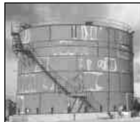
Boilermakers are building jet fuel tanks at the Anderson Air Force Base in Guam.
