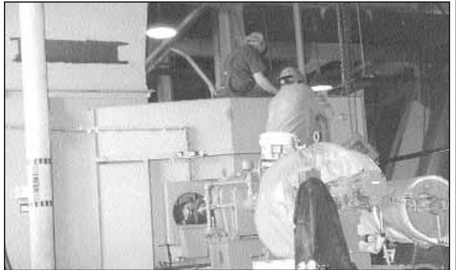
Local 193 members John Hambleton and Paul Zalenka install an induced draft fan, one of the last items to complete the 48-month project
