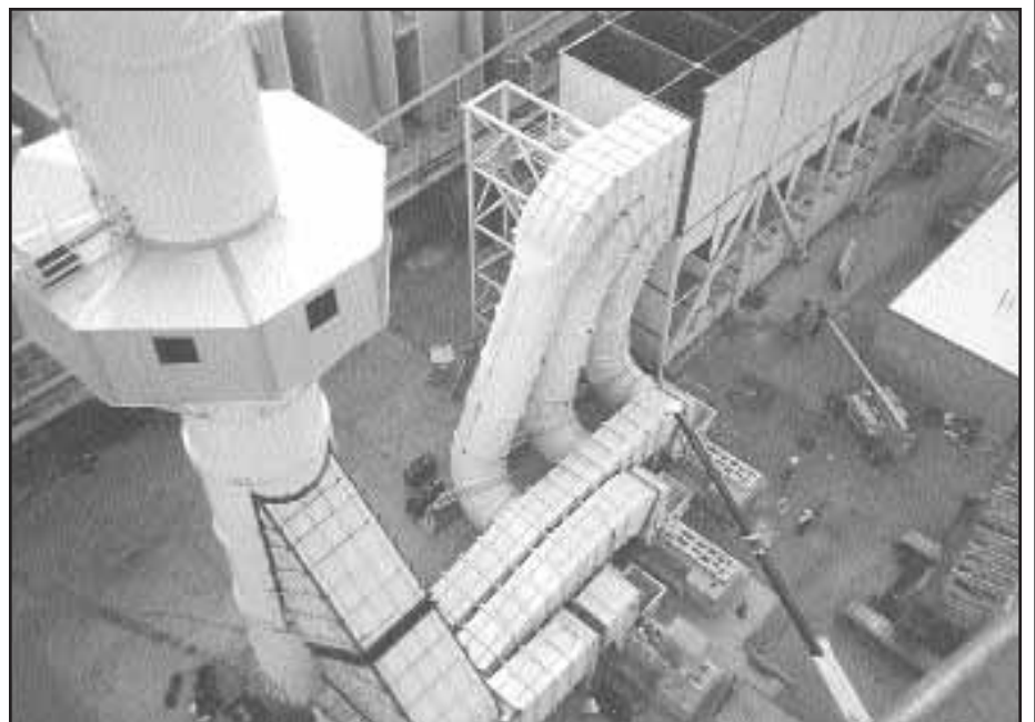
Local 242 members are building this recovery system for ABB Environmental at the Alcoa Aluminum plant in Eastern Washington.
