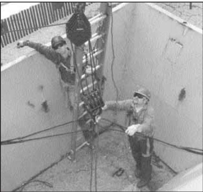
Great Lakes apprentices, Local 374's Clint Mace (on ladder) and Local 169's Richard Cowley, prepare to raise a hopper and set it on elevation during a rigging exercise.
