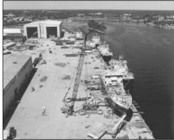
An overview of U.S. Coast Guard vessels under construction by Local 696 members at the Marinette Marine Corp. in Wisconsin.
