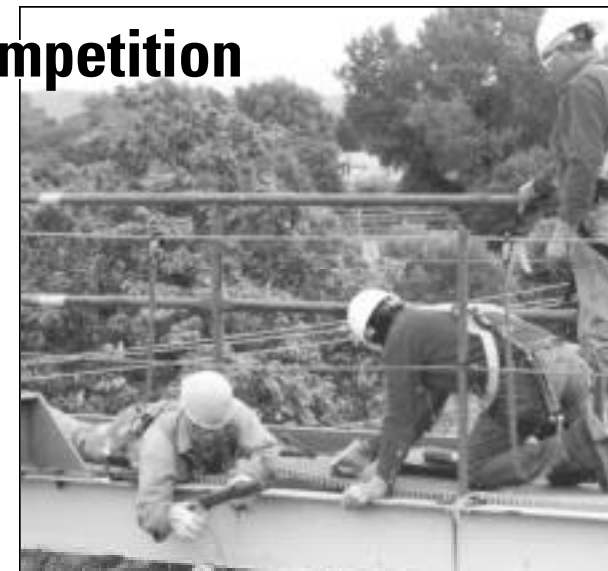
John Svensson of Local 502, Tacoma, Wash., installs softeners on a steel beam so he can attach a choker to hold a snatch block during the rigging competition. Observing are BNAP instructors John Standish and Carl Oliver.
