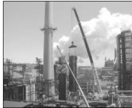
Members of Local 154, Pittsburgh, Pa., earned praise from Shenango Inc. for their work with American Boiler & Chimney on this dephenolization tower replacement.
