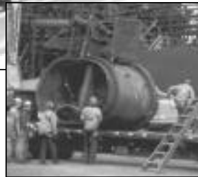
When this boom collapsed (top left photo), the 15.4 ton raw gas main valve pictured above fell 165 feet.
