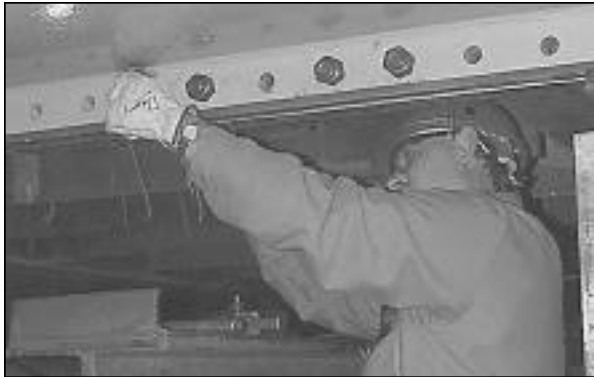
A Boilermaker bolts a waterbox to one of the new titanium tubed condenser bundles.
