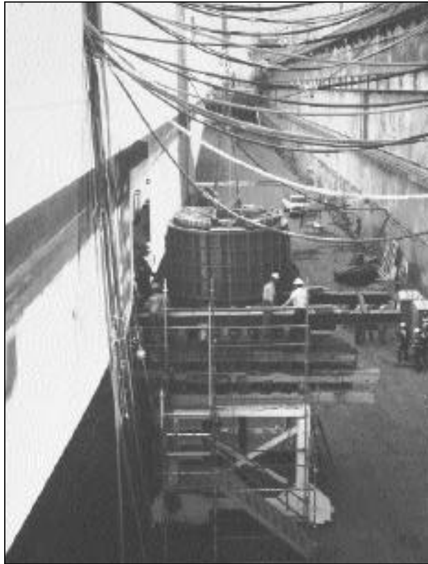
Members of Local 72, Portland, Ore., at Cascade General, work carefully to place a 43-ton, 8.5 megawatt replacement motor through a 25-foot by 30-foot hole cut into the side of the Rhapsody of the Seas ' hull. Once inside, it was skidded into position. Photo by J. M. Schif fhauser, ©1997.
